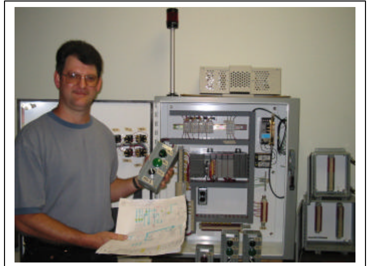
Mr. Neil Slabaugh is shown here with a PLC based control cabinet and remote operator station.
